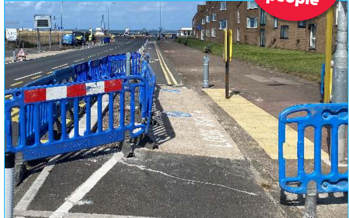
The cycle lane on Harrison Drive has cost at least £181,000 but still isn't right. The Town Hall 'forgot' to include the tactile paving to warn blind and partially sighted people of the kerb.
